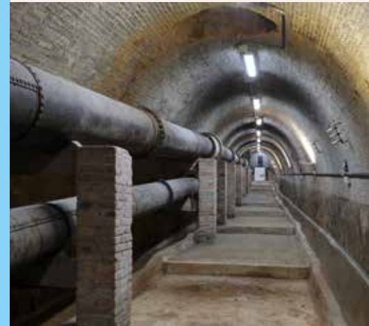
Interior of the tunnel connecting the houses in Trinitat Vella and Trinitat Nova. © MUHBA/Manuel Cohen
