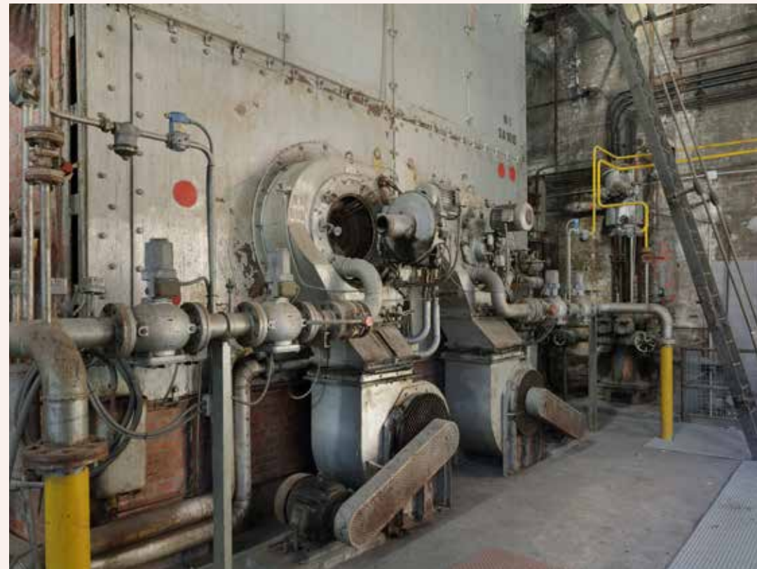
One of the Babcock & Wilcox boilers inside the room. © MUHBA/Manuel Cohen
